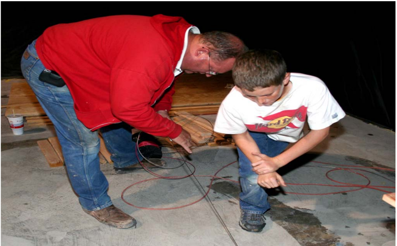
Tom Jones and Adam Jones prepare to thread electrical wire through floor conduit
