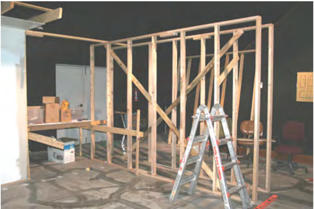
East side view of the new twin walls constructed Saturday, January 28. These two walls will support the temporary return loop bench work. Later they will support parts of the East Tower vicinity in the Amarillo yard on this side and the Canadian yards, including the wagon bridge and the railroad bridge on the west side. The upper level will support Umberger on this side and Texico, NM on the west side.
