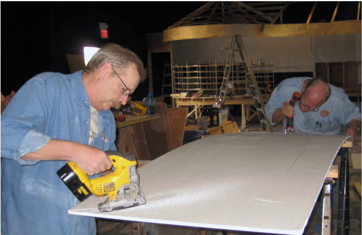
A week has passed since the installation of the backdrop behind the Helix. Earl Carrell and Virgil Doyle cut out the final piece of sheetrock for the ceiling over the backdrop and the approach to Canyon.
