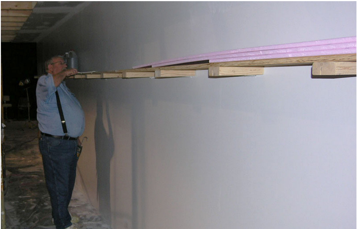
The Canyon-Umberger segment of track, supported by shelf brackets, runs along the South Stud Wall. The segment is actually straight here; the curve is the result of parallax. Virgil Doyle is attempting to hold the track to keep it from curving as the picture is made.
