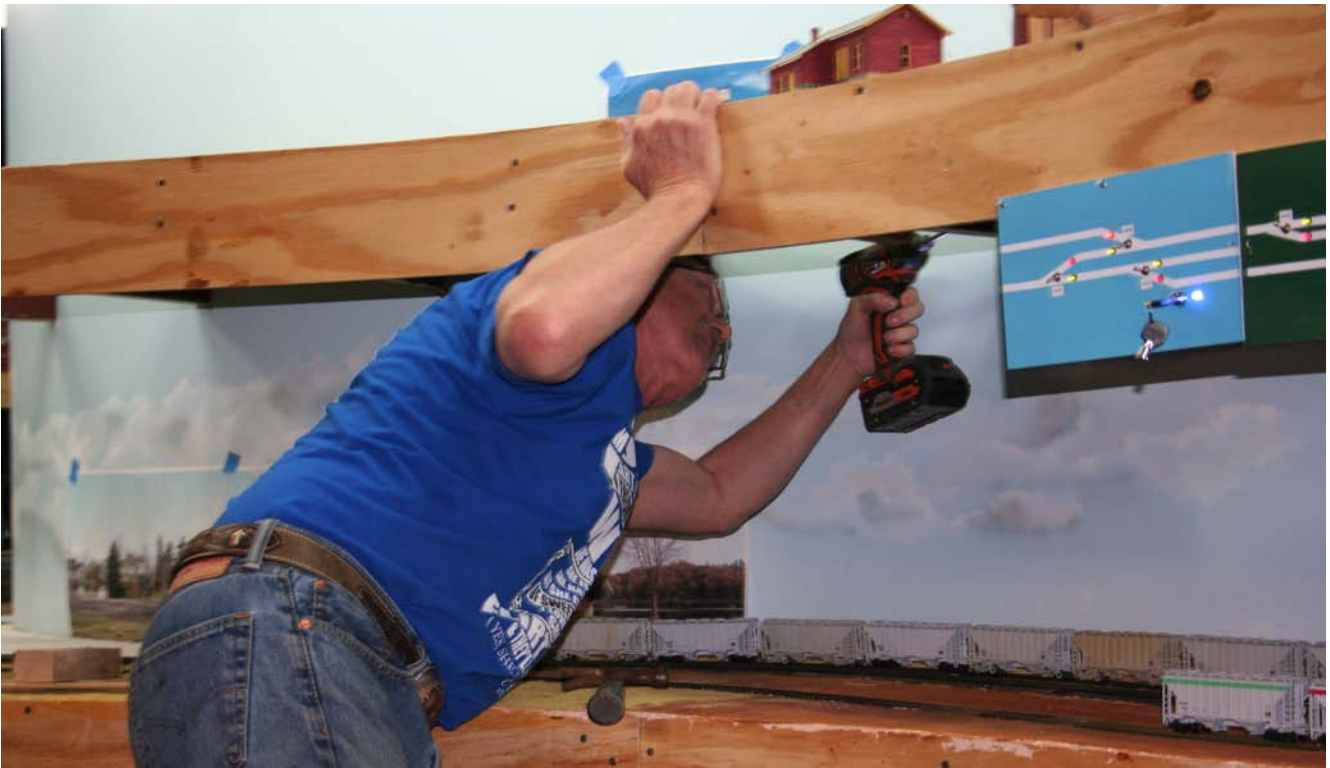
February 22, 2020: Chris Mitchell installing support for extension of decking on the upper level at Texico above Canadian.
