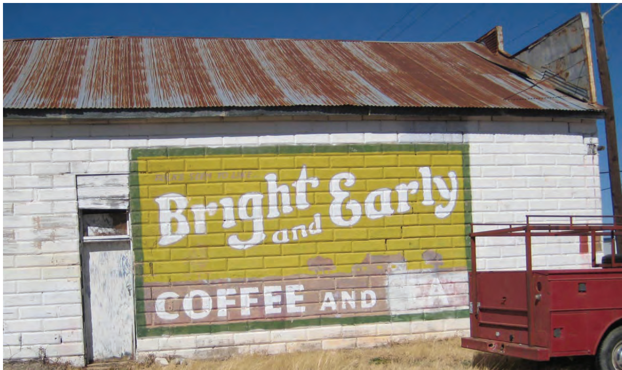
Rising Star, TX. Check the rusting on the roof! These signs were once found everywhere in Texas. 2-18-09.
