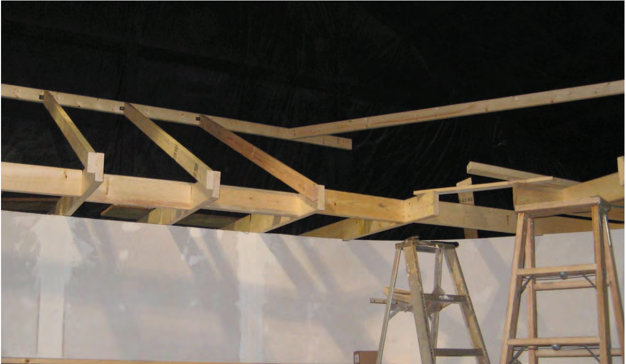
This is the way it looked before installing rafters at Southeast corner on 2-19-09
