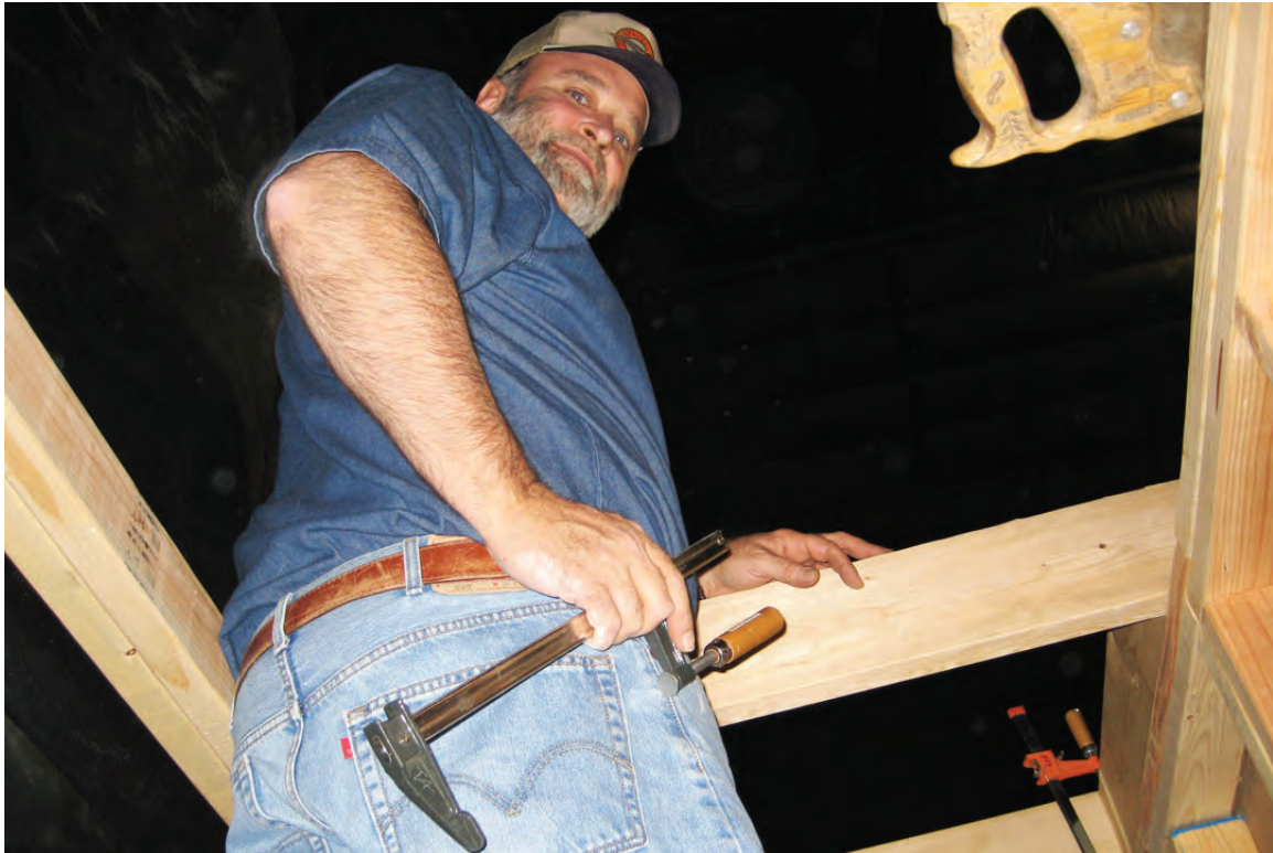
Jerry Michels ready to clamp a joist in place. The brace helps space the joists.
