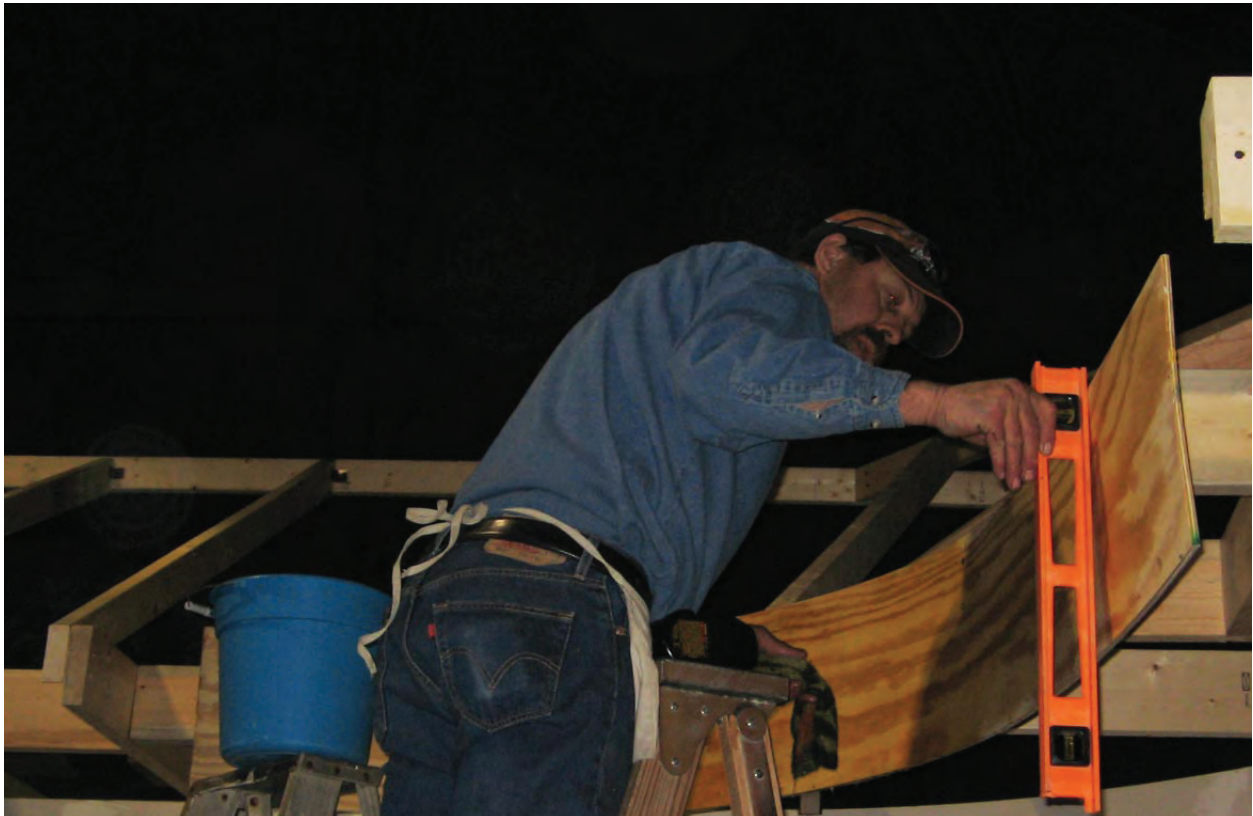
Tracy squaring up Tracy's Bend in the fascia after rafters were installed. 2-19-09
