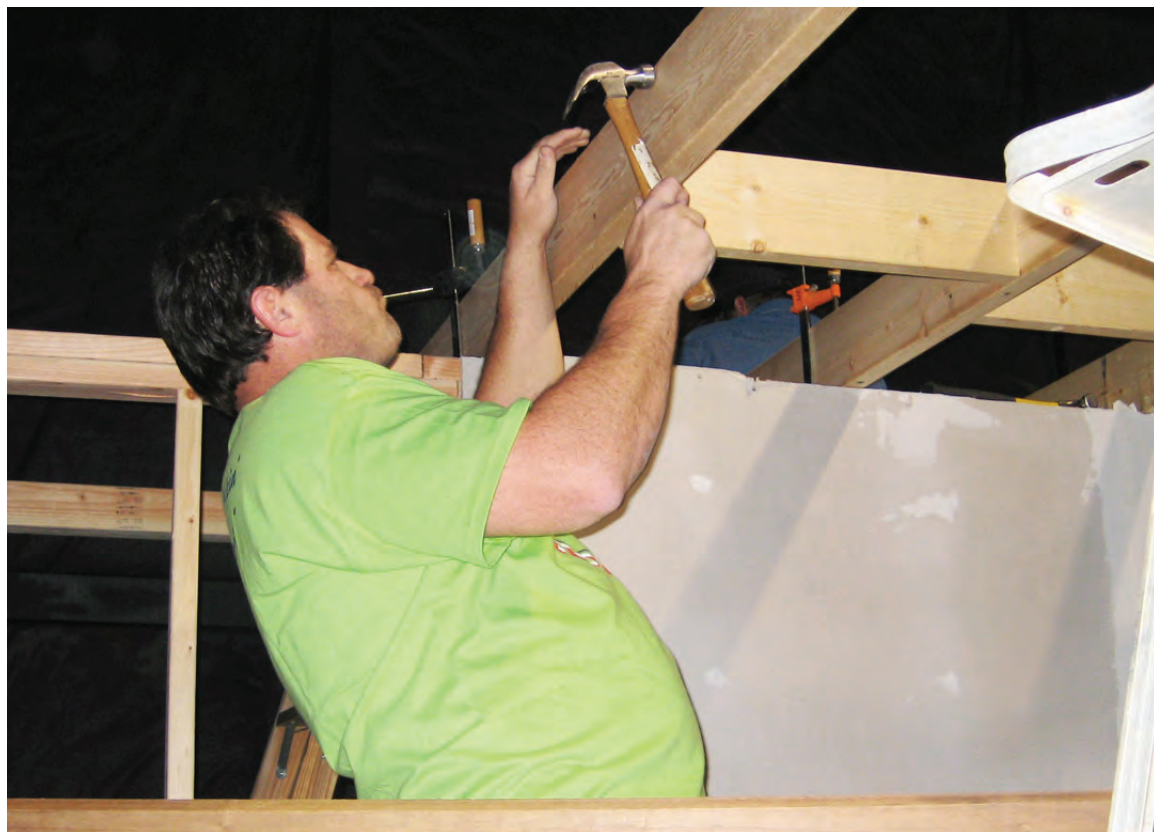
Carter Osborne nails a brace in place. The braces keep the joists from rotating.
