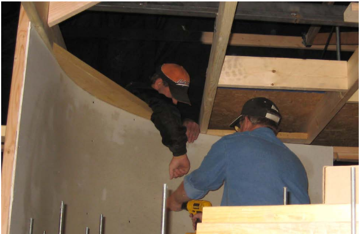
Tracy Ball holds the sheetrock next to stringers while Earl Carrell sets the screws on the last part of the first section of the curved backdrop over the Helix.
