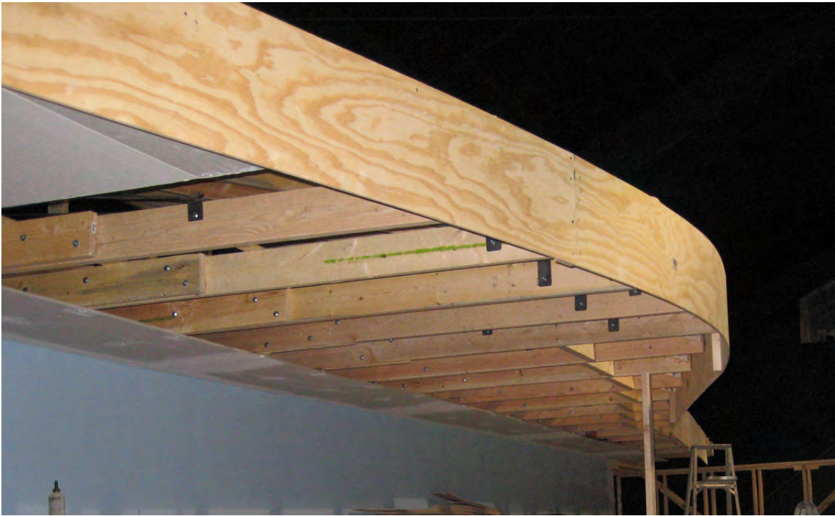
View from underneath showing area needing sheetrock over the Amarillo Yard..
