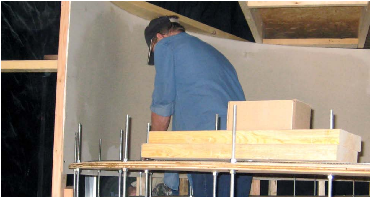
Earl Carrell, helped by Tracy Ball, Virgil Doyle, Bob Roth and Jerry Michels behind the scene, fastened the first corner of the curved, 1/4-inch-sheetrock backdrop around the top of the Helix.
