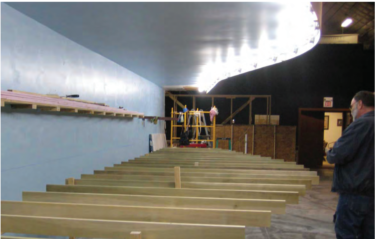
Amarillo Yard Bench and newly-installed lights. Everyone, including Jerry Michels, is proud of the accomplishment.
