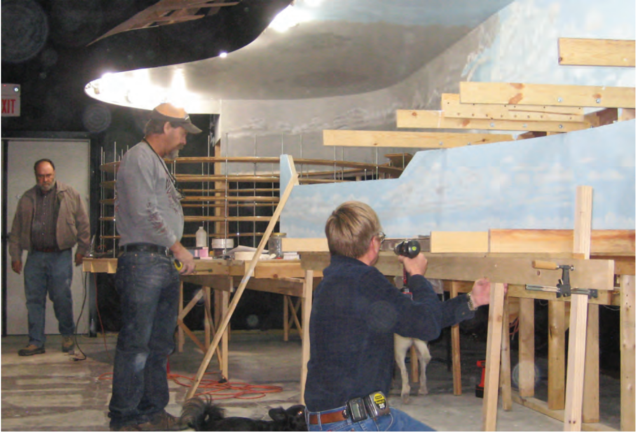
Jerry Michels, Tracy Ball and Bob Roth build framework for the lower level bench.
