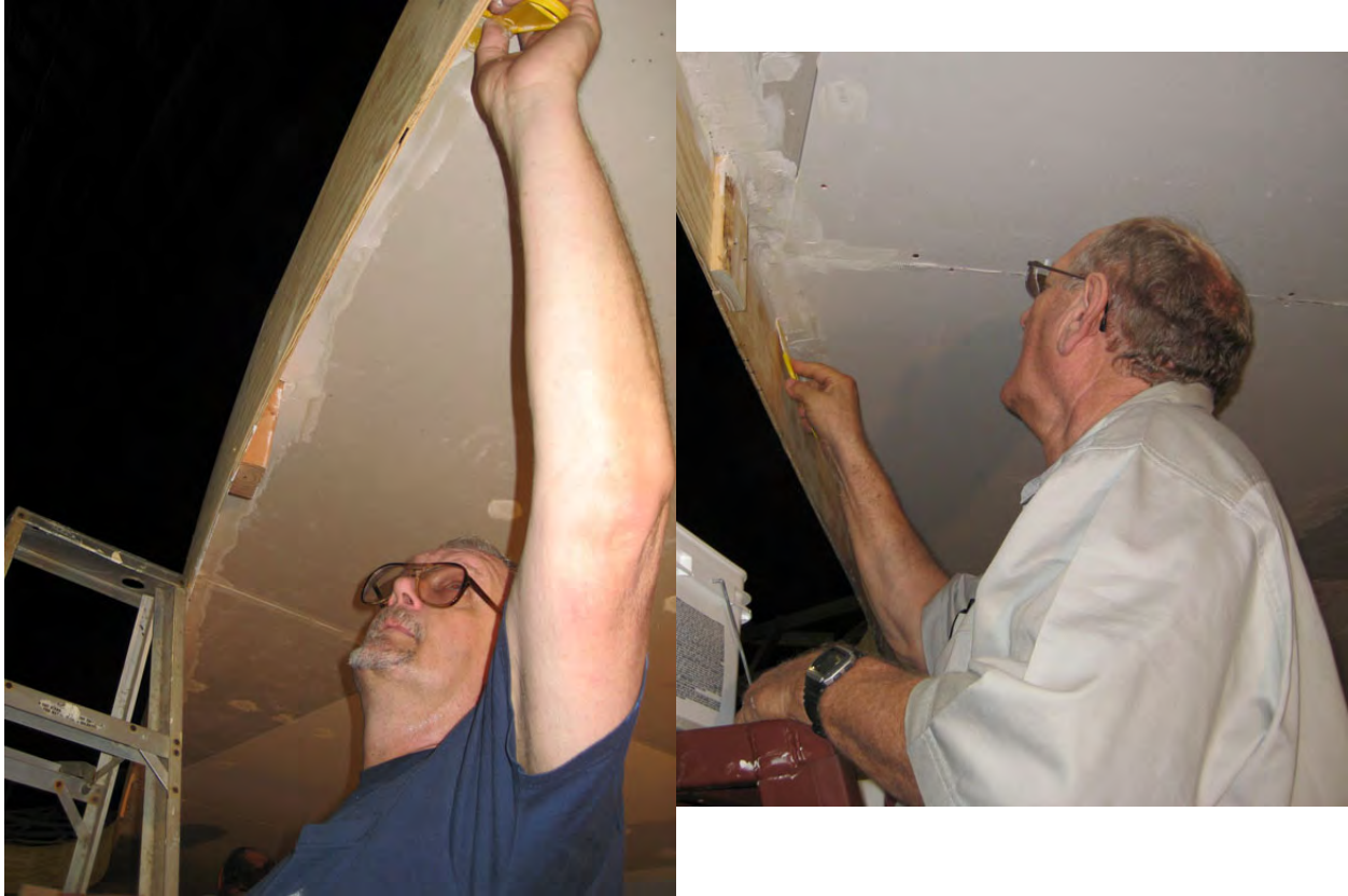
Dave Jusiak and Virgil Doyle continue to fill in the joints over the Amarillo Yard.
