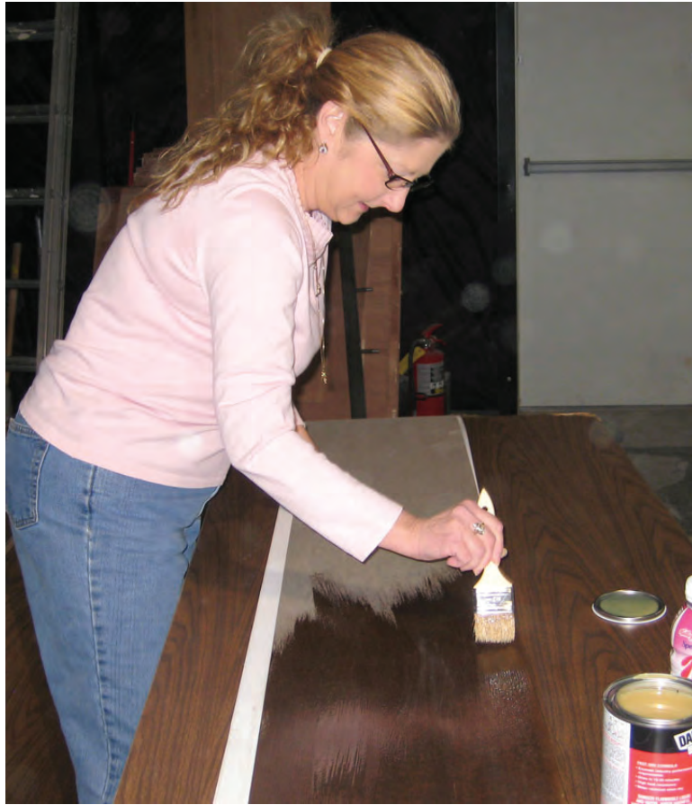
Reva applies contact cement to a panel of black formica before Tracy hangs it on the fascia.
