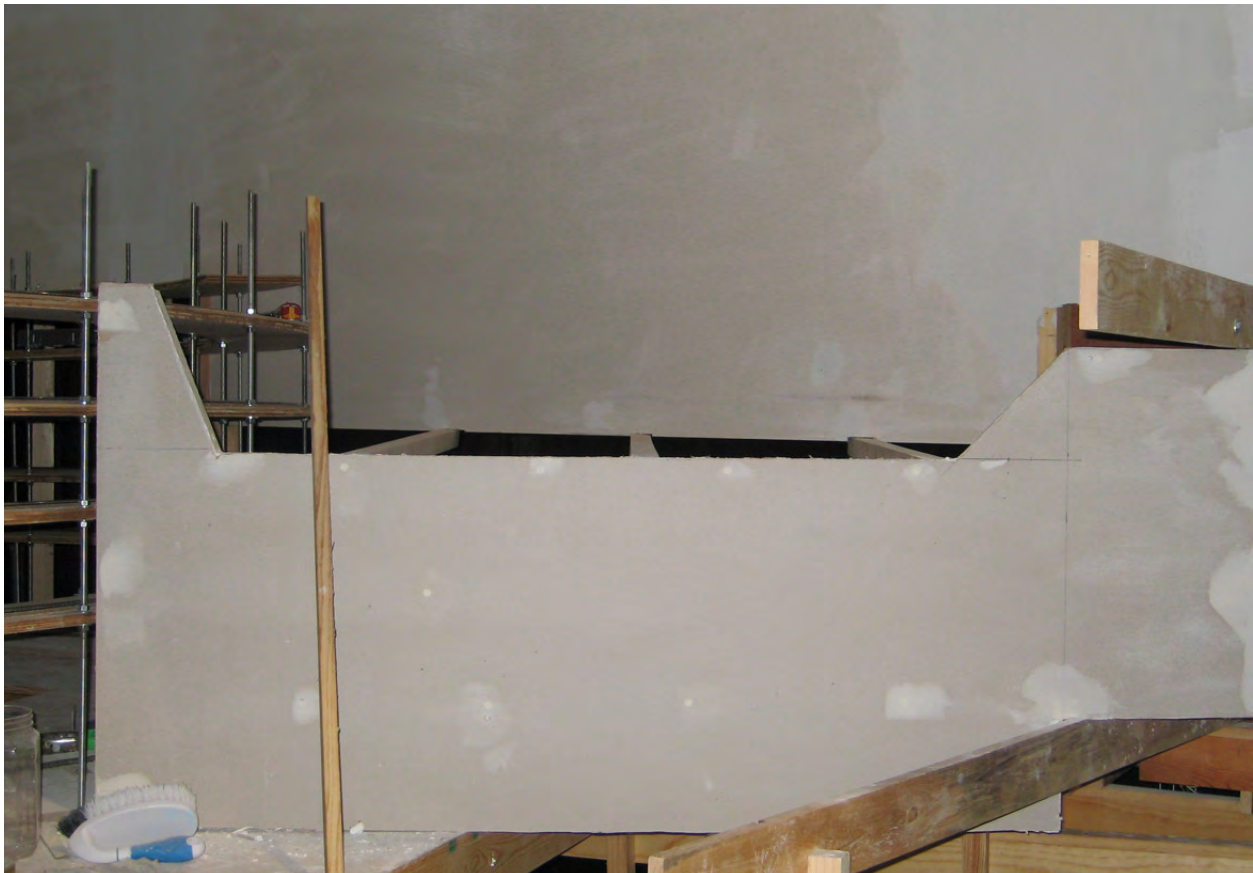
Transition area between Helix and the upper and lower benchwork. The upper level will enter from track near the upper end of the leaning board. The lower level will enter from track near the blue spot on the lower backdrop.
