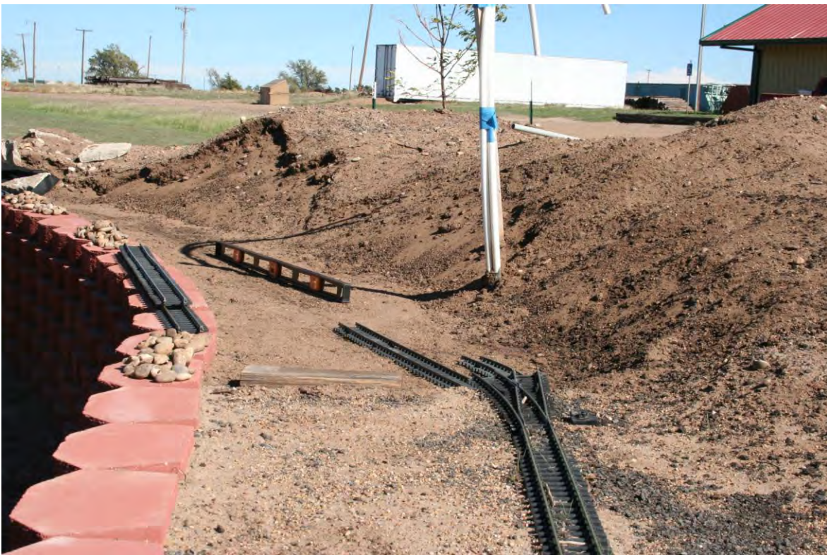
Garden: Effort showing to level the bed for the track on the North side of the garden.
