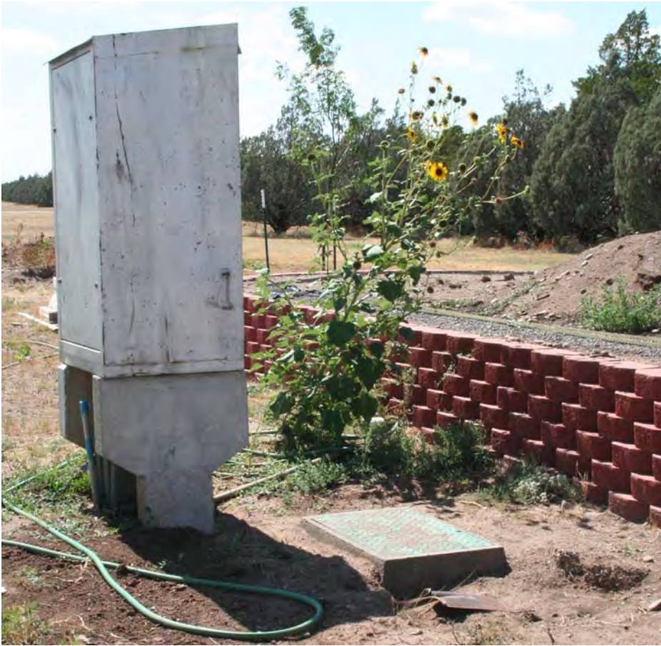
New valve box housing the sprinkler system control valves for the garden.
