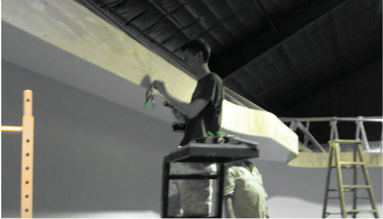
Brian Jansky makes a minor correction in the alignment of the fascia panels. Virgil Doyle is not far behind in filling in the gap between the fascia and the ceiling.
