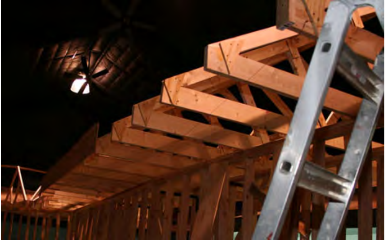
Fascia on the North side of the Peninsula. It lacks over 8 feet in length to close the gap.
