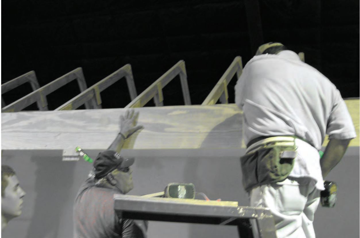
Brian Jansky, Joe Calvin and Jerry Michels are working from the right lowering the fascia. They are approaching the last panel.
