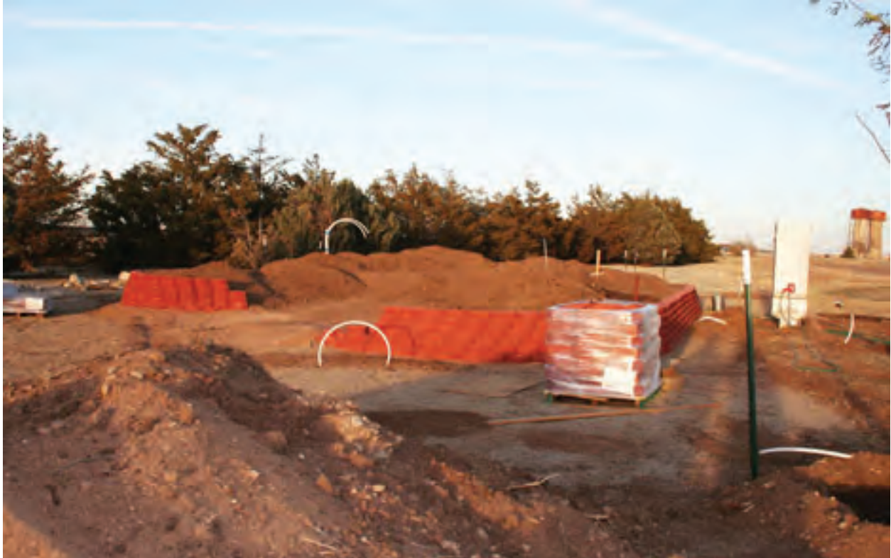
The gap in the wall which allows the tractor to get inside and shape the dirt pile. Several more loads of dirt will be added before the rest of the stones are put into place and the Wall completed. The snow made it almost impossible to load dirt at the dump site.
