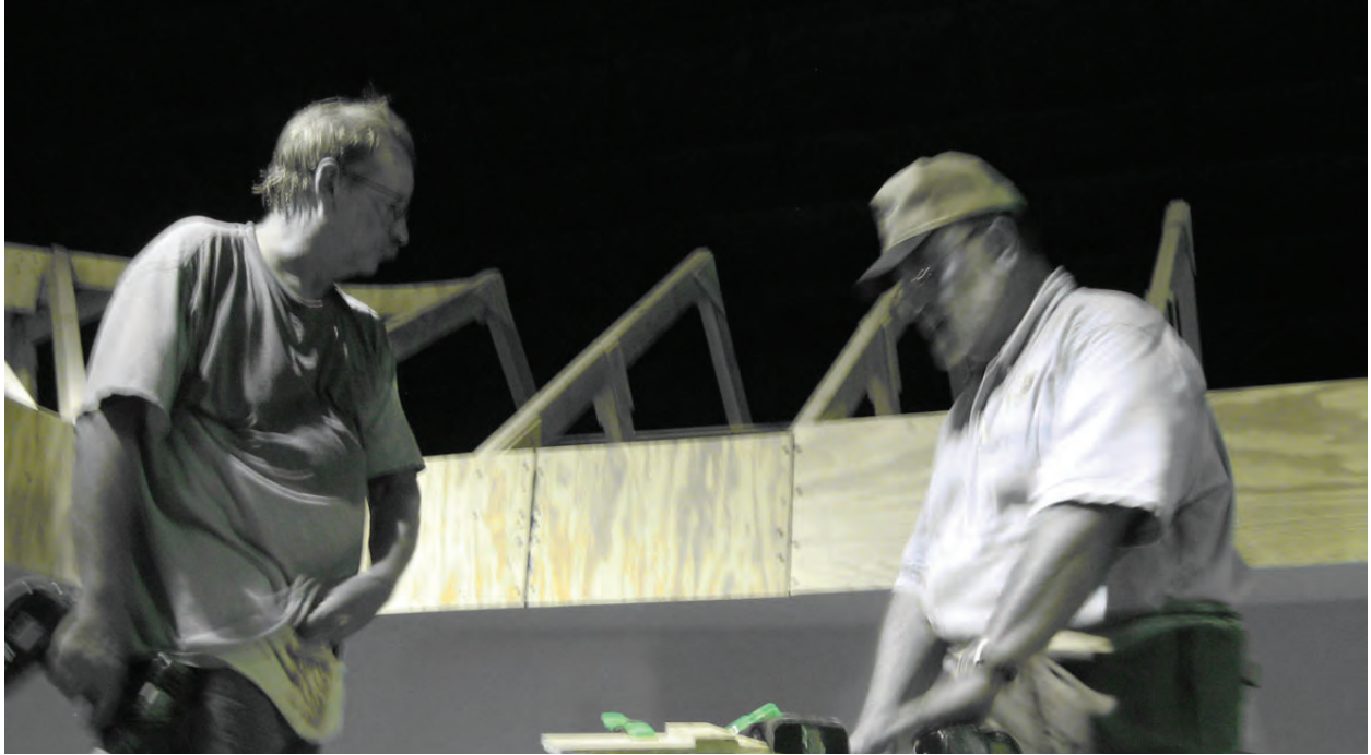
Earl Carrell and Jerry Michels have just installed the last panel of the lowered fascia. The black and white appearance is due to the light from the overhead lights. It is mostly green.
