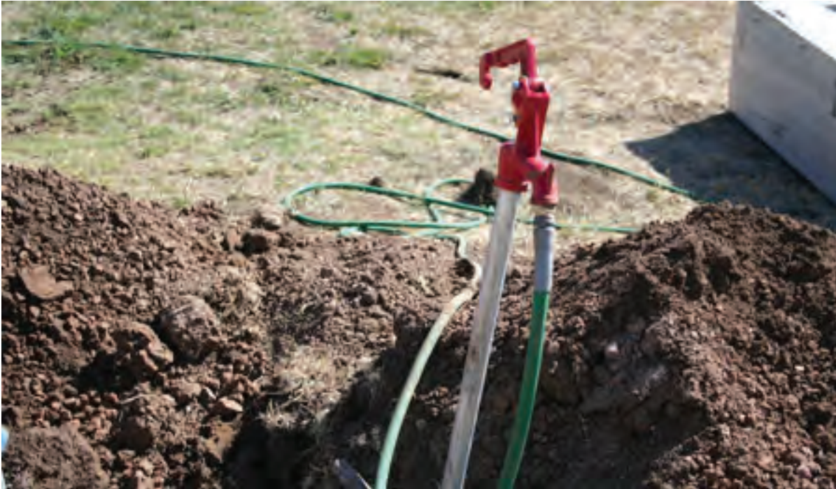
The frost-free faucet has water connected to it. It will stand beside the Electrical cabinet.
