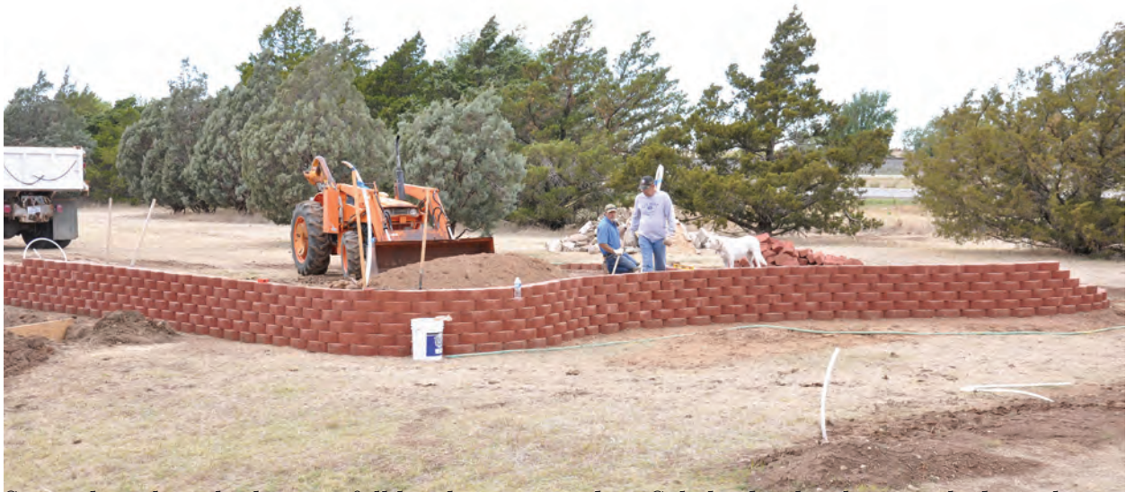
Stones have been built up to full height on two sides. Caliche dirt has been packed into base of wall. Photo by Jerry Michels.
