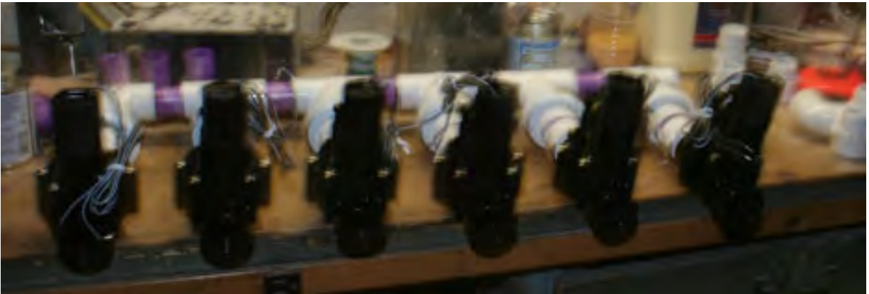
Electric control valves installed in manifold
