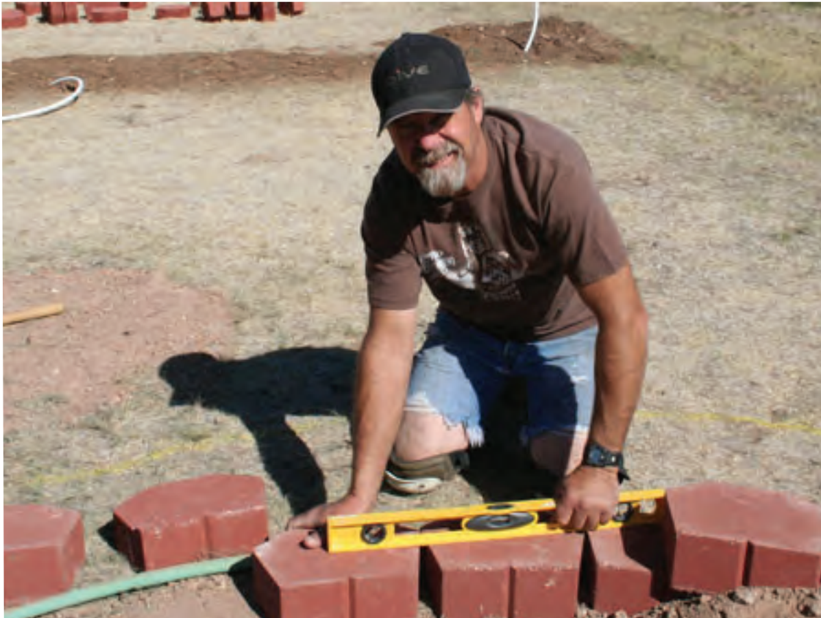
Tracy placing and leveling the first level of stones. The water hose defines the border.
