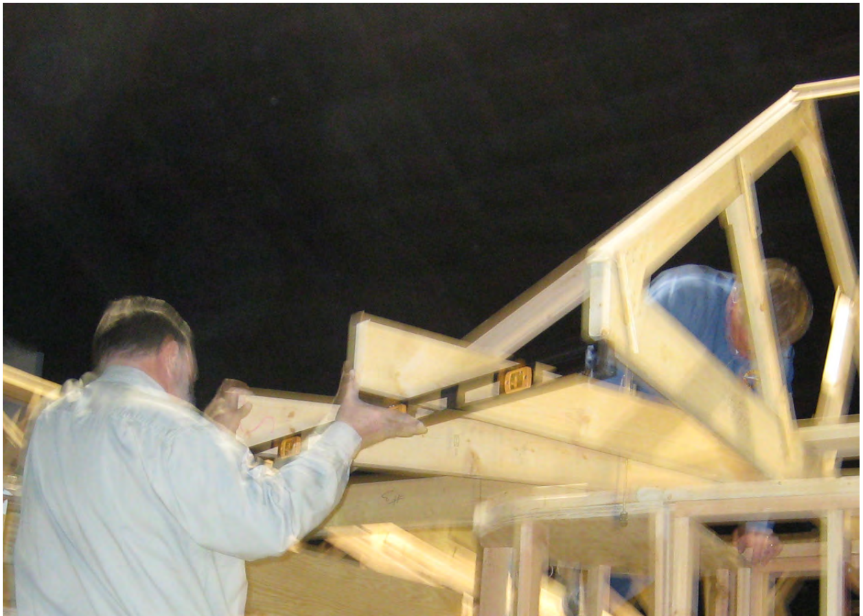
Jerry and Bob working on the girders at the end of the peninsula.
