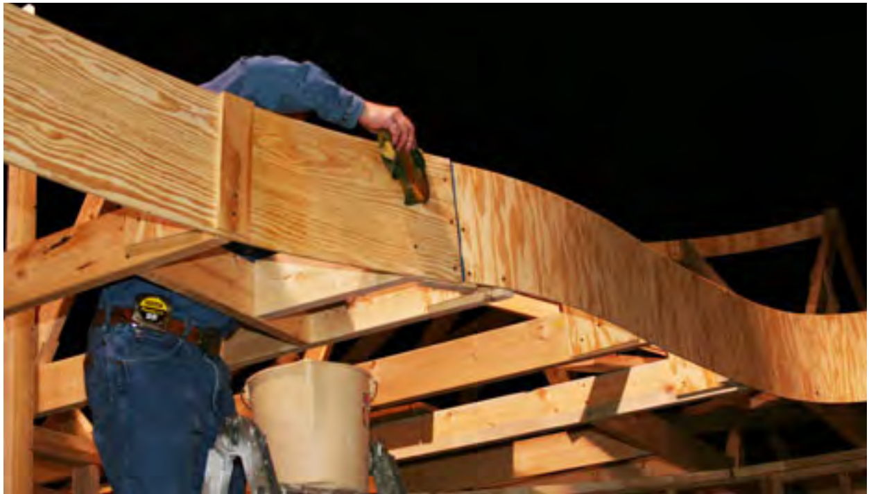
Bob Roth has to wet this segment down so it will curve with less strain.
