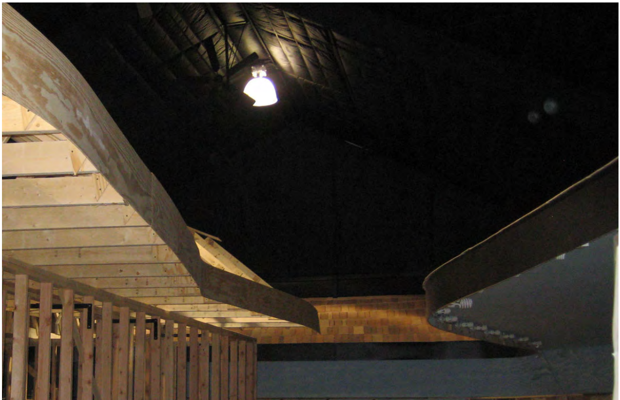
Fascia boards installed over Pampa yards (left) and finished fascia over the Amarillo yard (right). Note the sweeping curves.
