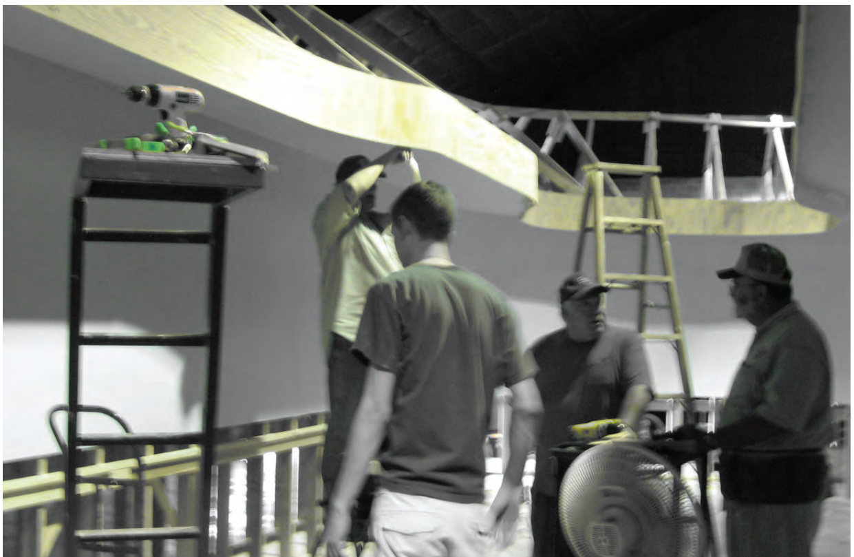
Virgil Doyle filling gap,, Brian Jansky, Joe Calvert, Earl Carrell and Jerry Michels breathing a sigh of relief that the fascia is completely lowered. And it was HOT!
