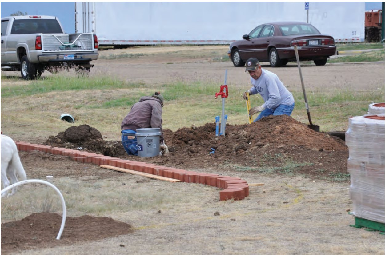
Tracy and Earl preparing ditch for setting electric cabinet posts. Photo by Jerry Michels.
