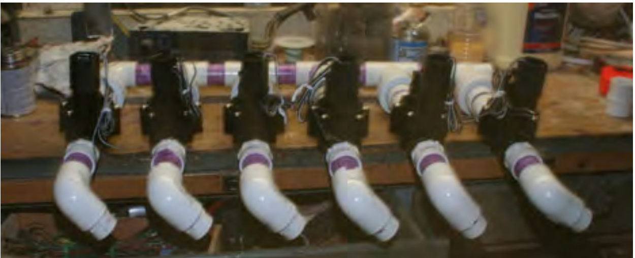
Els and adapters installed in finished manifold
