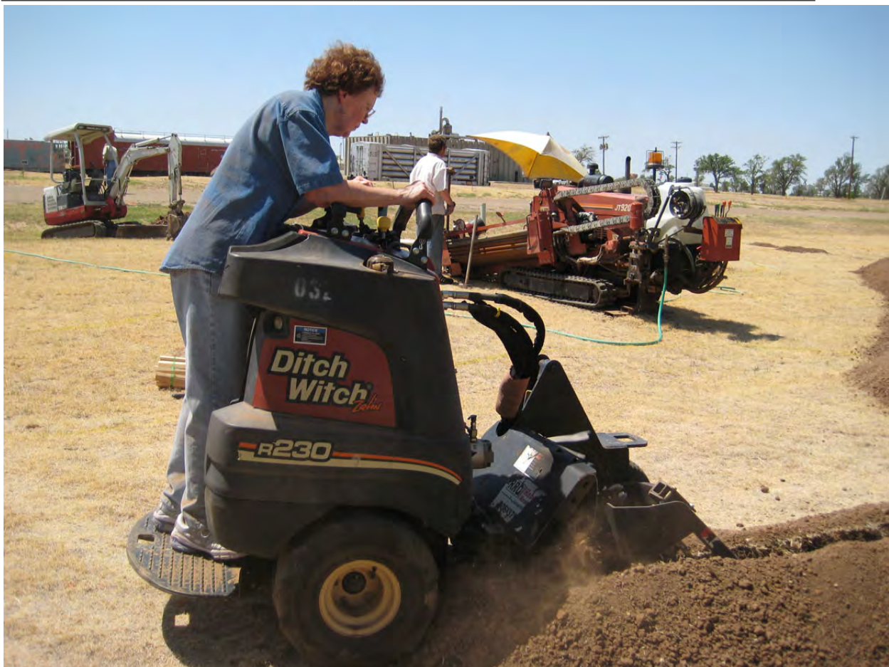
Paula Young runs the ditcher while Dave Hebard and helper bore hole under the pavement. After Tracy got off work, he ran the ditcher.
