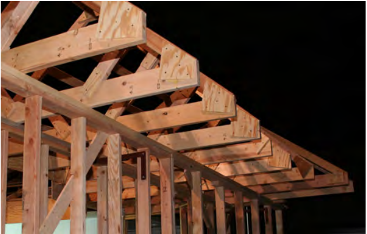
One of the last steps, the South end of the outside West wall.
