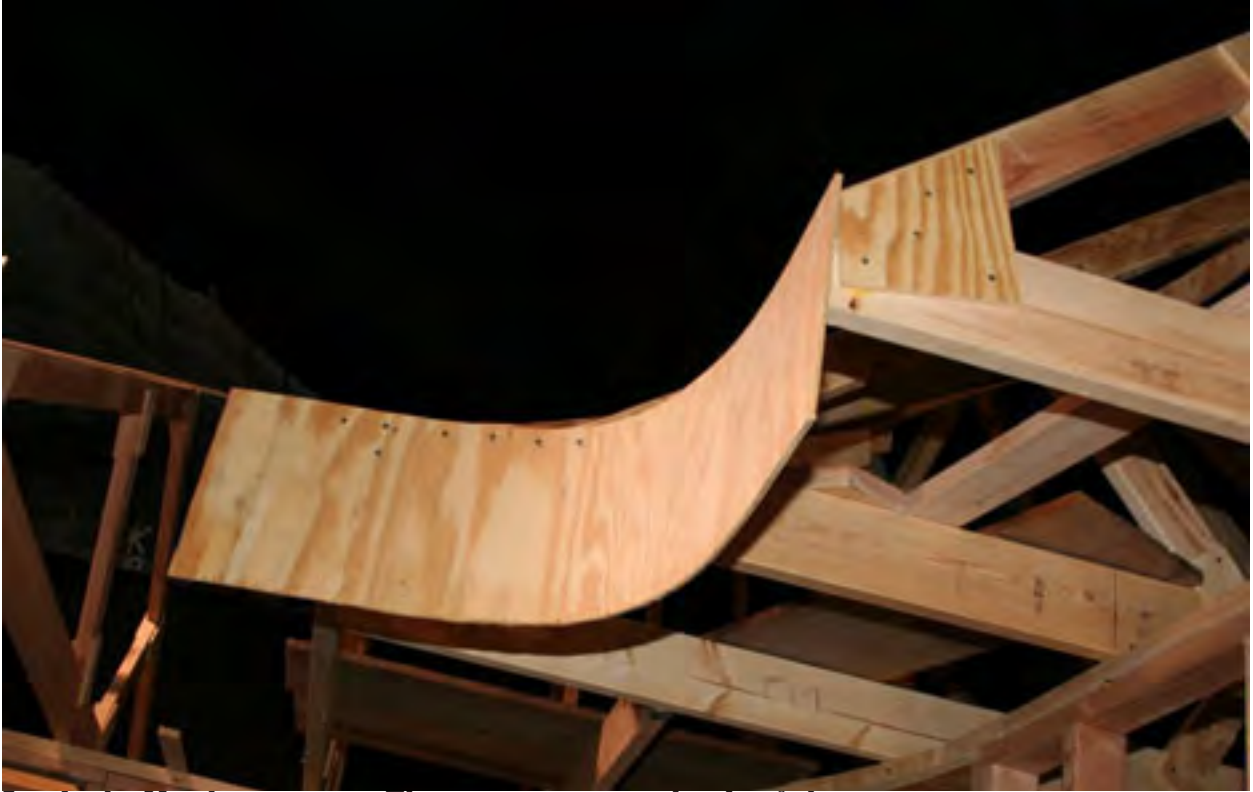
Inside the Northwest corner. There are gaps on each side of this piece.
