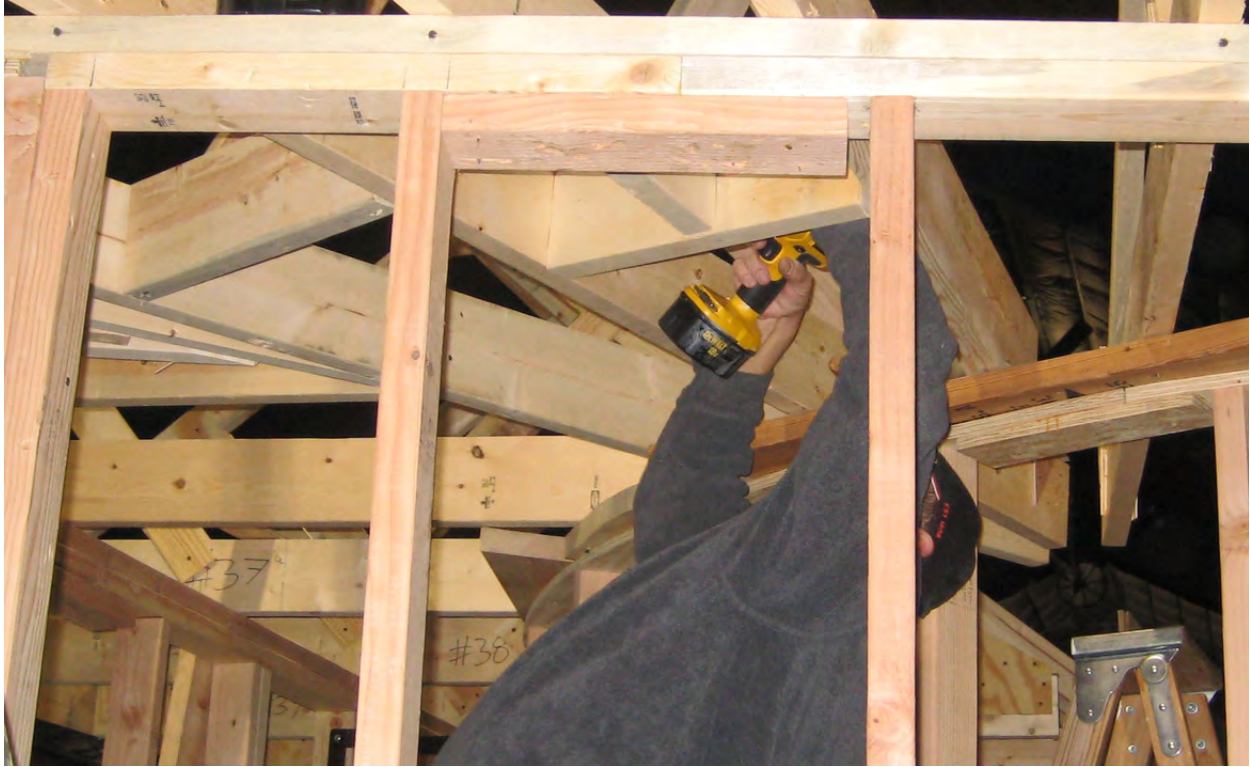
Earl in the middle of the framework connecting the ends of the girders.
