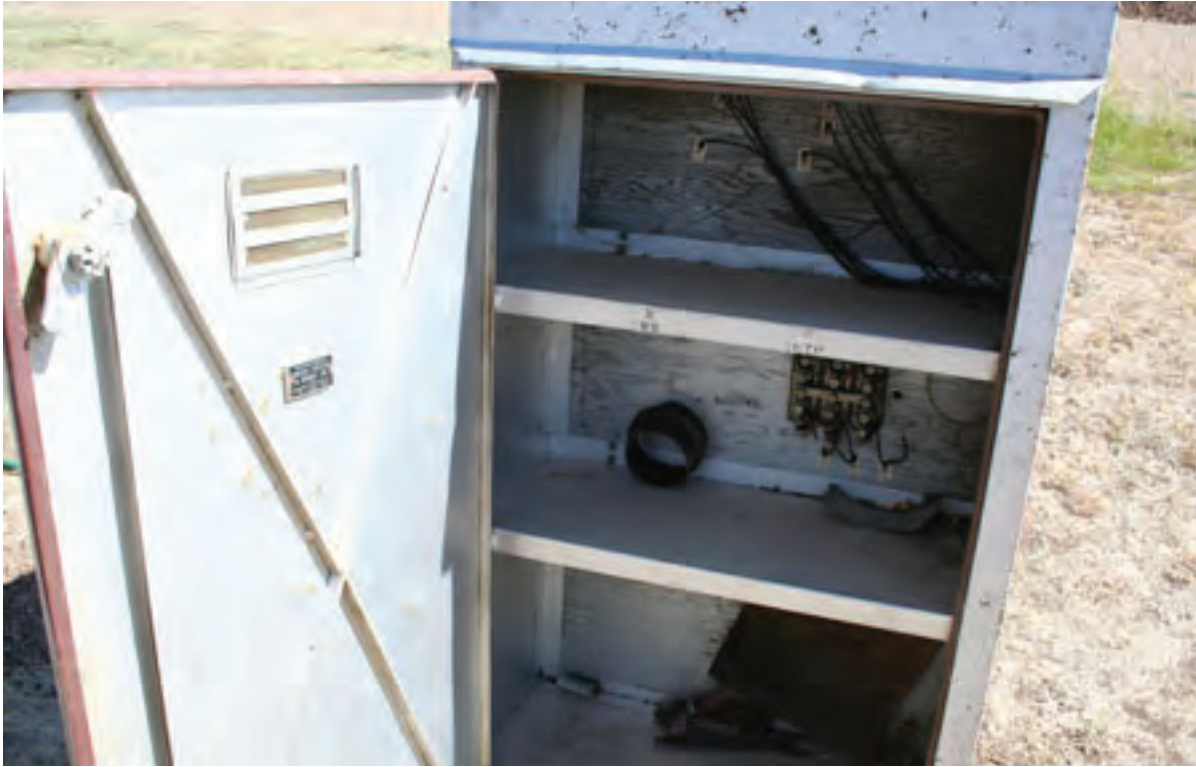
The instrument Box open. A breaker box and other accessories will be stored here.
