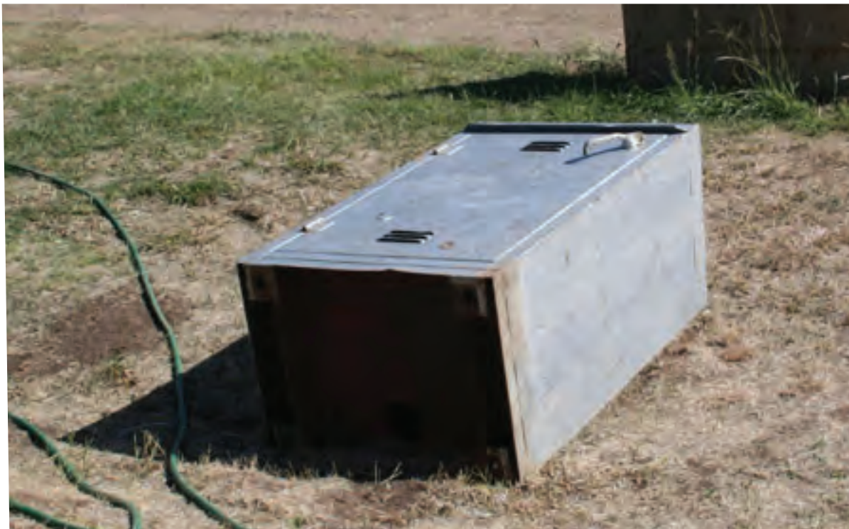
It is difficult to see the four holes in the bottom of the electrical cabinet. You can see the rectangular plates in each corner which reinforce the holes.
