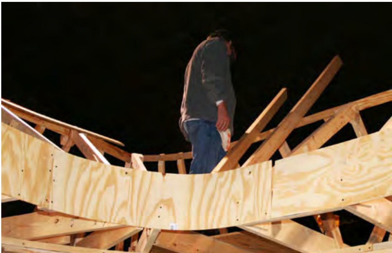
The SE corner gap is closed. Earl Carrell is using the backside to measure for inside rafters.
