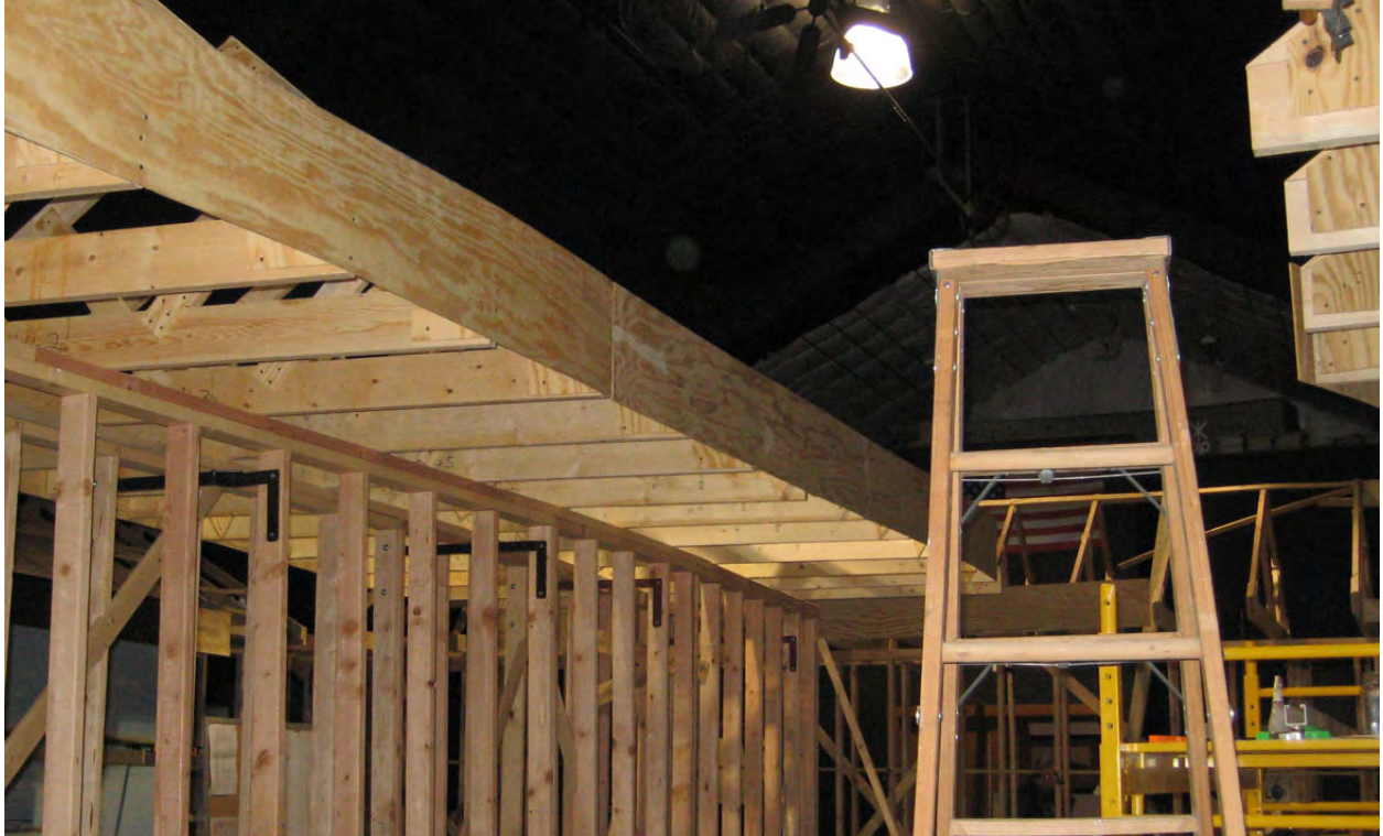
Fascia boards have been installed in several places. These are on the North inside wall.
