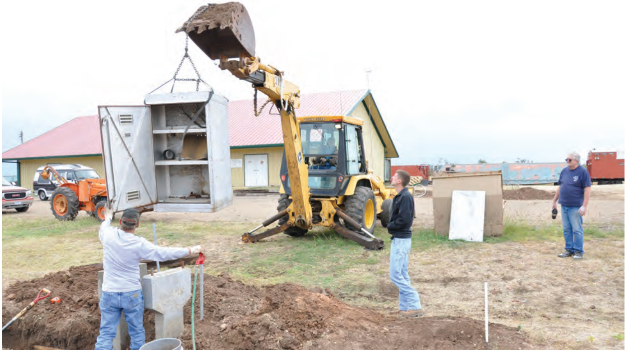
Earl and Tracy lowering Electric Cabinet onto support posts. Brian and Dave are supervising.
