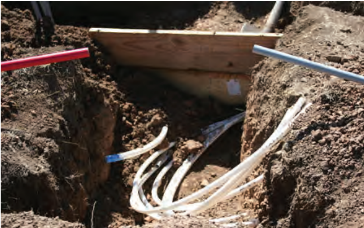
The hole for the manifold. Tracy will cast in place a concrete frost box. The incoming water line is to the left and the six circuit water lines to the right. The control wires from the timer will also come in here.
