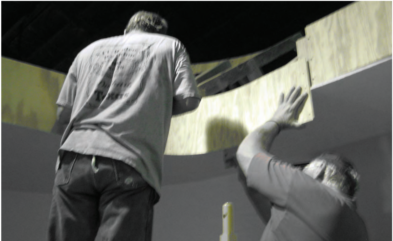
Earl Carrell and Joe Calvin line up the next-to last panel. They are working from the left.
