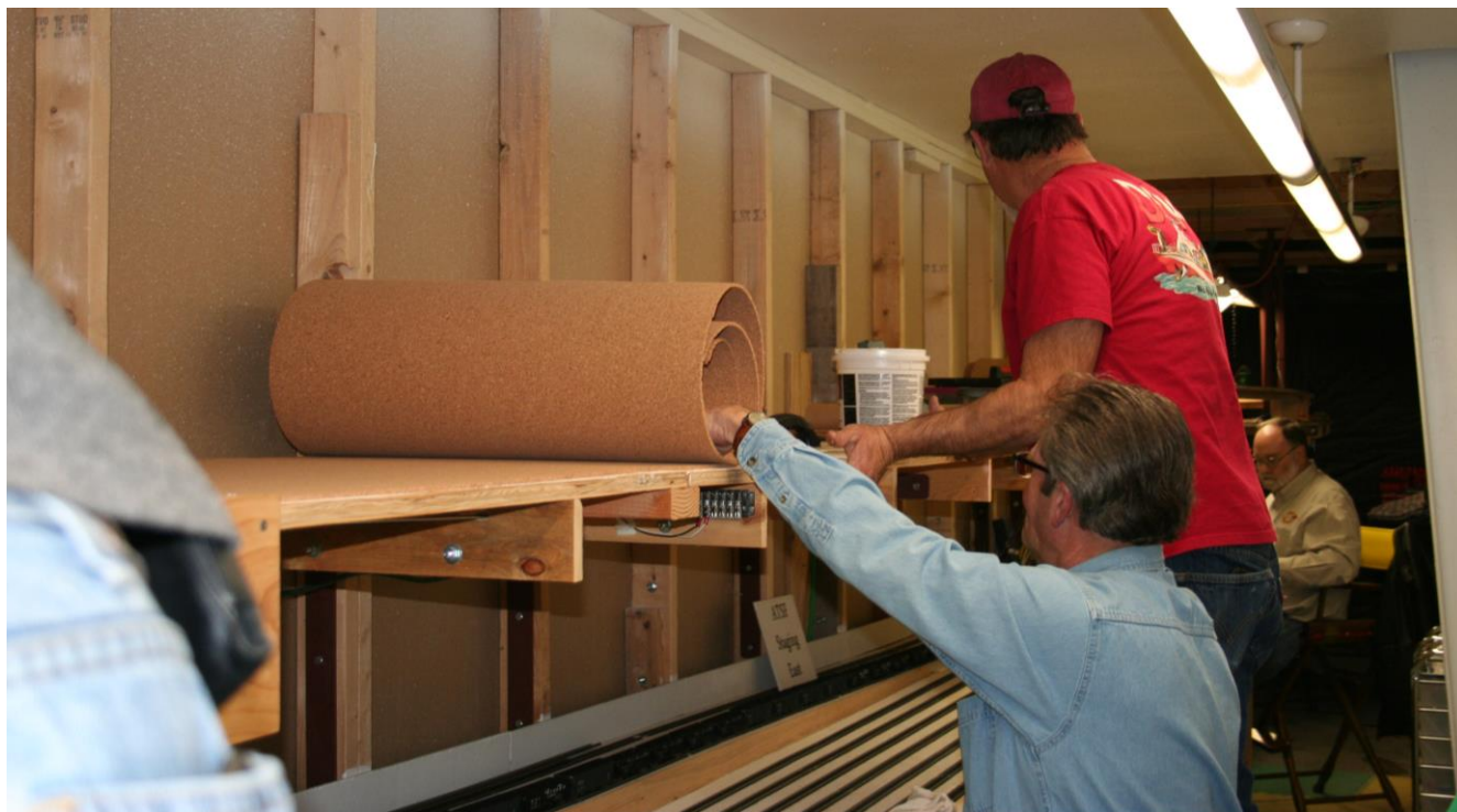
January 25, 2018: Bruce Carter and Tracy Ball laying-out cork for the upper level Staging Yard.
