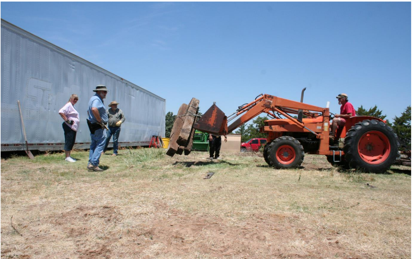
June 9, 2018: A team effort was made to clear the area on the East side of the storage trailer to make room for another storage trailer.
