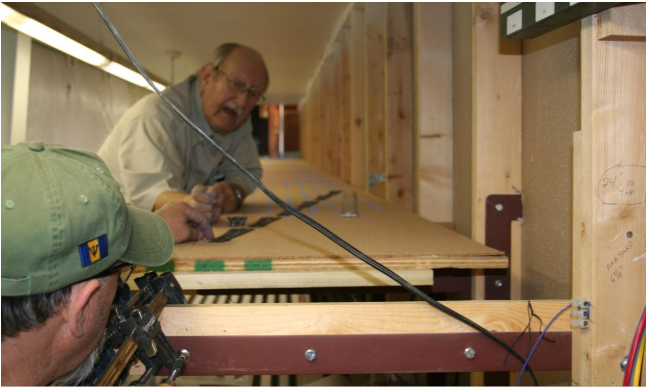
March 24, 2018: Tracy and Virgil laying-out switches for one end of the upper staging yard.
