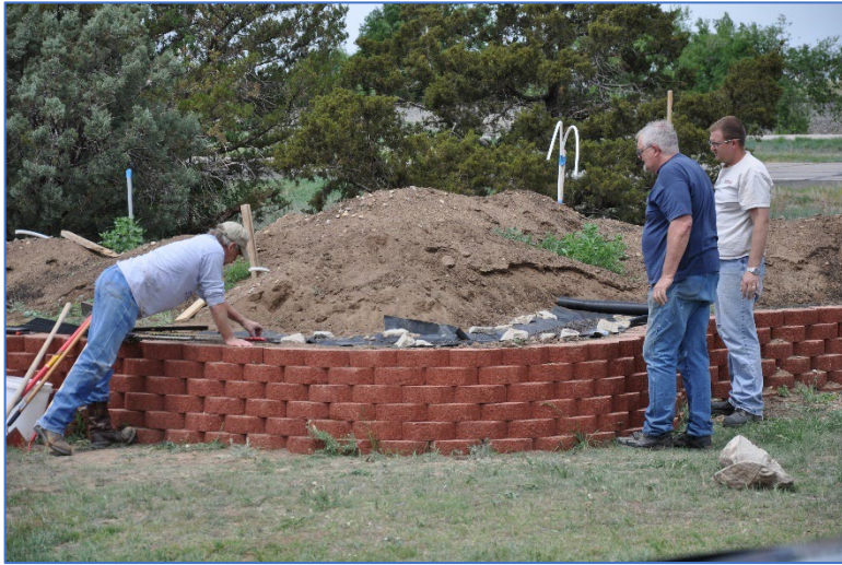
Earl Carrel, David Jusiak, and Craig Jusiak work on the roadbed of the PPMGRwy to make sure the track will be laid on a smooth surface.
