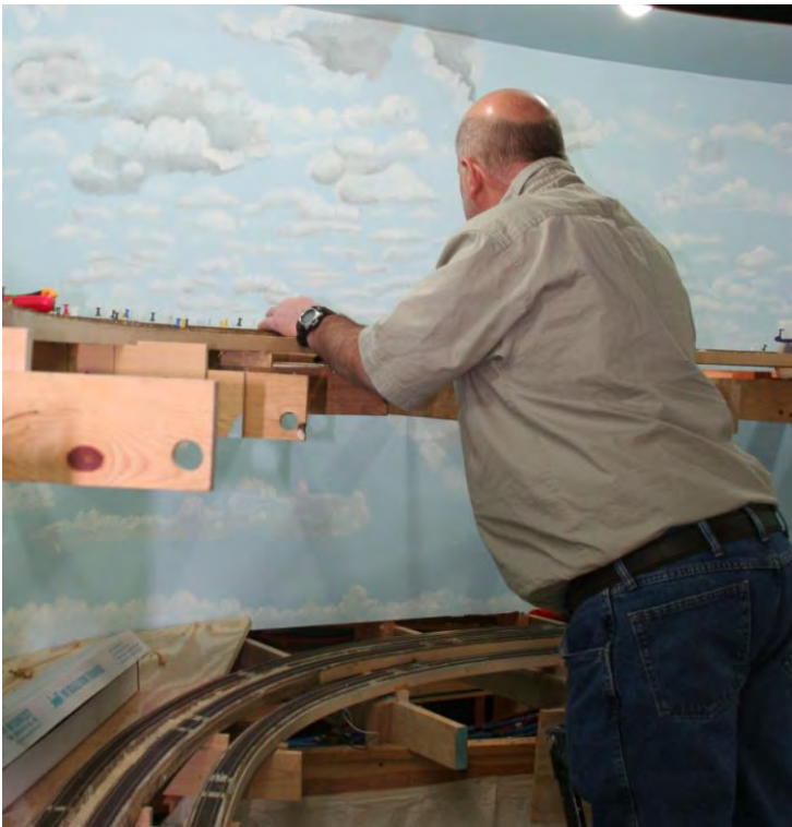
Guy Pigg installing cork roadbed on the completed spline on the upper level.
