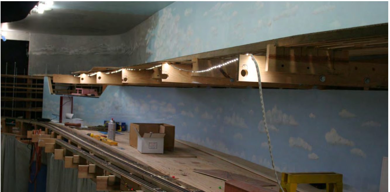
February 27: LED strip lighting acquired for lighting Zita on lower level below Canyon. LED strip is just laid over the upper level supports in this photo.
