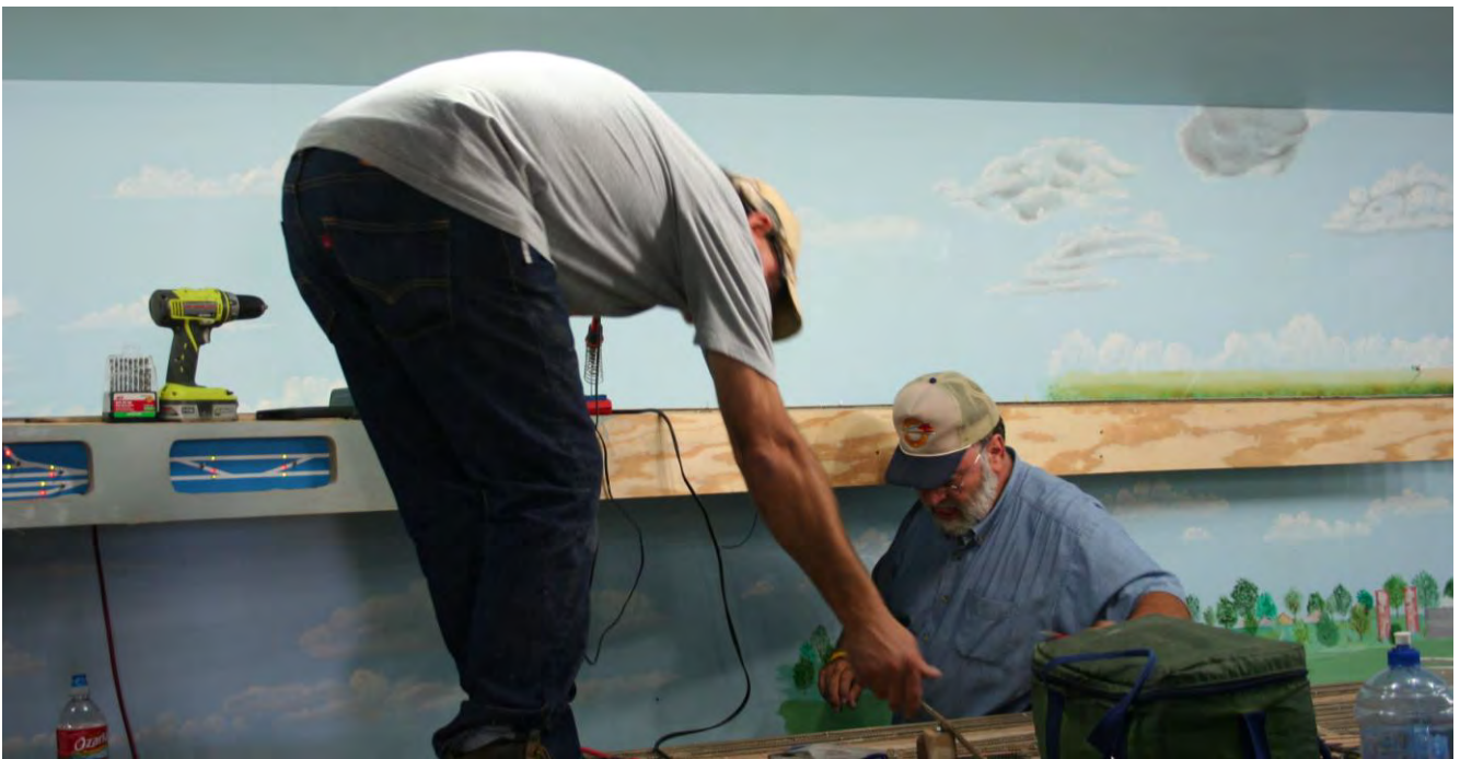
Aug. 23: Tracy Ball and Jerry Michels installing power drops on upper level tracks.
