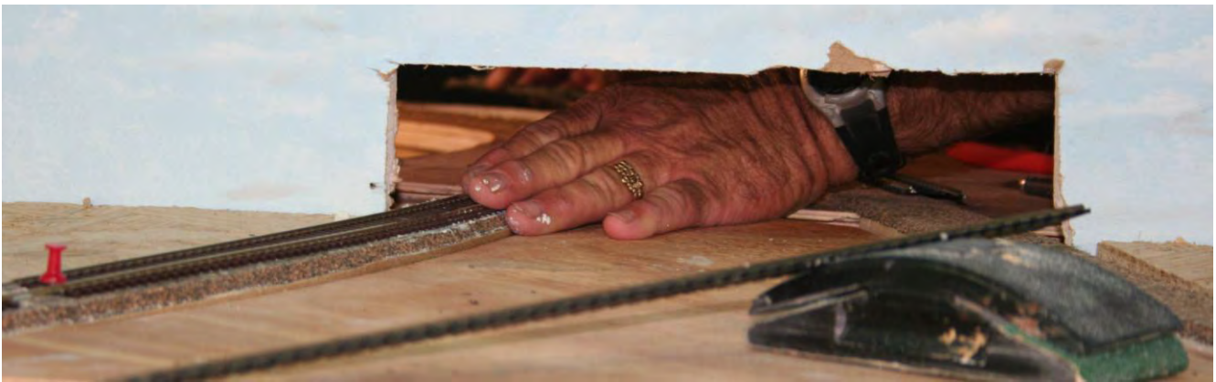
May 24: Tracy Ball is laying the track around the East leg of the wye at Canyon behind the wall.
