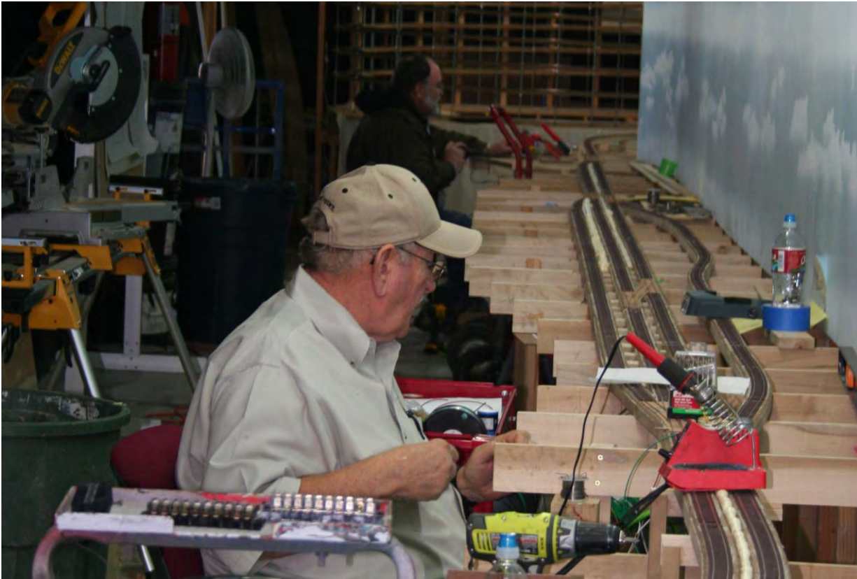
February 8: Virgil Doyle working on the temporary control panel for the turn-out at the East end of Miami (foreground) while Jerry Michels works on track power bus for side tracks at the West end of Miami.
