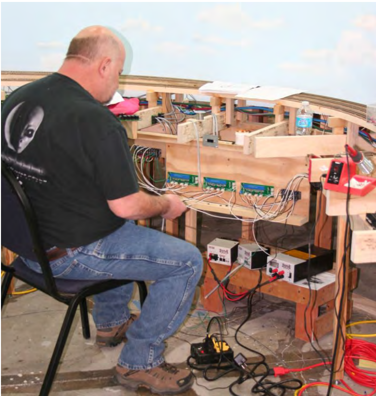
February 27: Guy Pigg working on installation of track power boosters near Cuyler.
