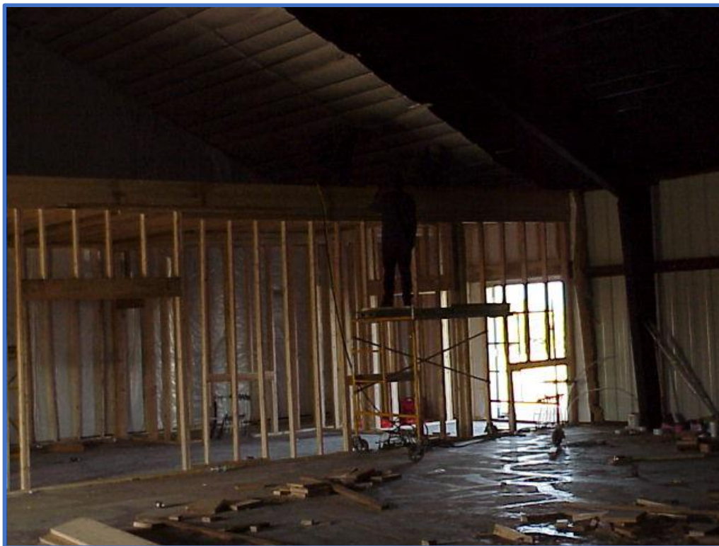
Top. A view looking northeast from the layout room toward the main entrance into the 25x50 ft. meeting room. Bottom. Looking south from the meeting room. The restroom aisle at left, the entrance to the kitchen at right. At far left is the entrance to the layout room.
