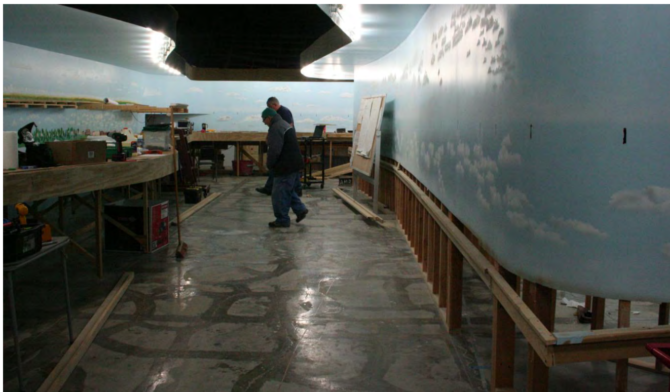
Pampa side of peninsula: Saturday, January 12, David Jusiak and Joe Sweeny move boards out of the way from around the base of the bulletin board. Clean-up effort was started an hour earlier.
