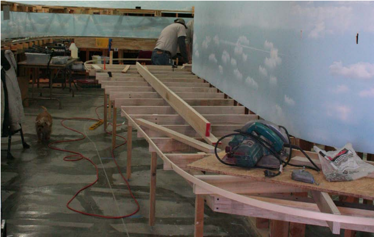
Bench work around the East end of the layout between Pampa around the corner at the far end of this bench and Miami to the right. Tracy Ball is working on the far corner. Note the use of the spline strip to achieve the smooth rounded corner.
