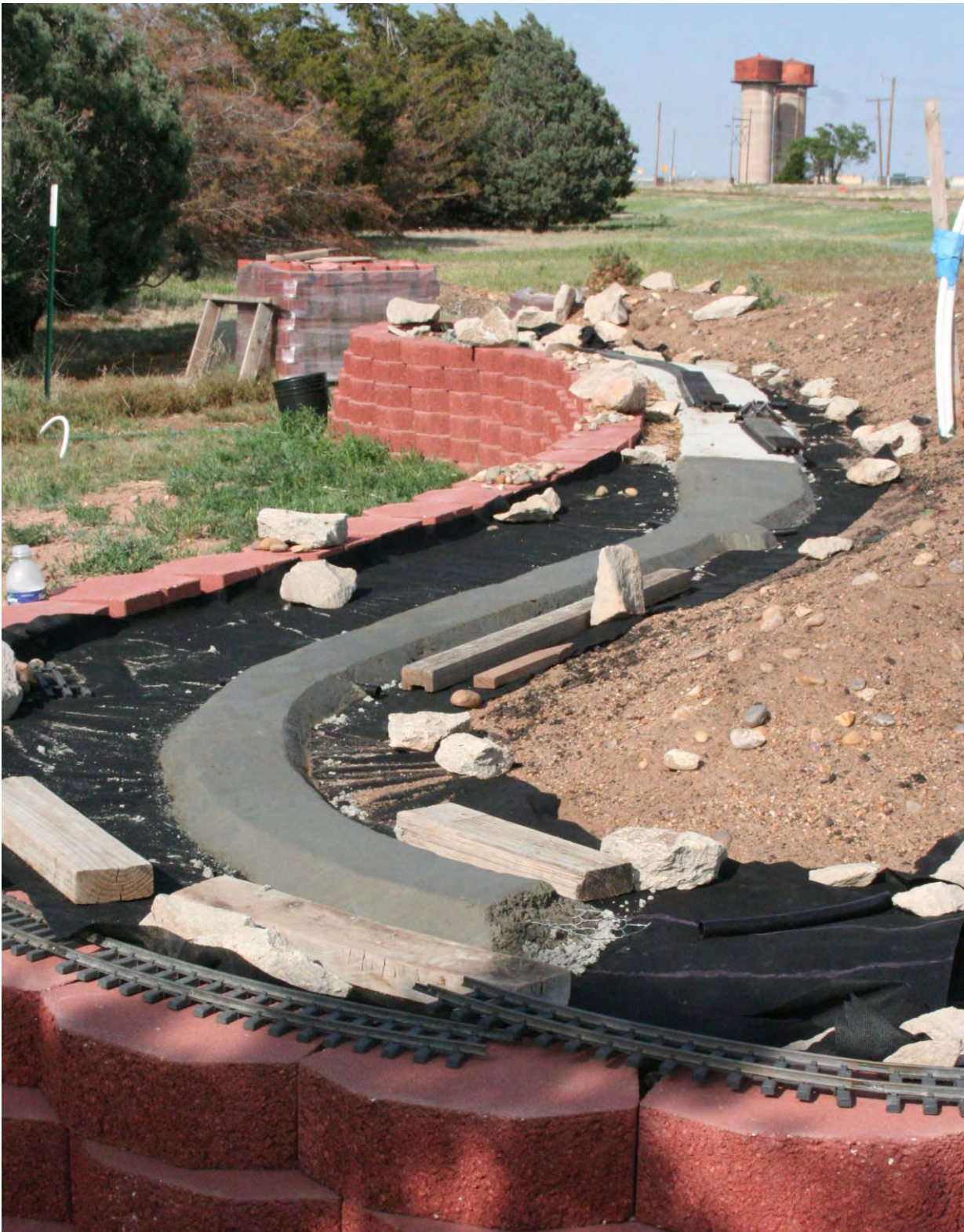
Freshly laid roadbed on the North side of the Phillip Pratt Memorial Garden to support the track. Next step will be installing the track on the roadbed after the roadbed is extended further.
