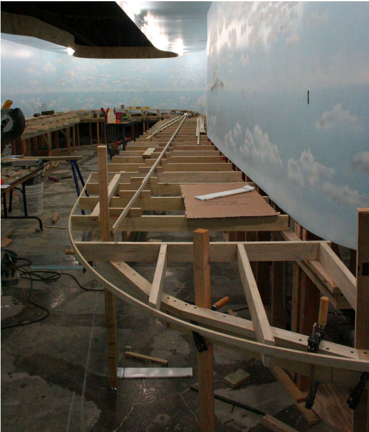
First leg of the spline sub-roadbed extending down the length of Kingsmill. Cuyler is located at the far end and Panhandle is on the opposite side of the aisle. This was the status of construction on the layout at the end of the day on January 26, 2013.
