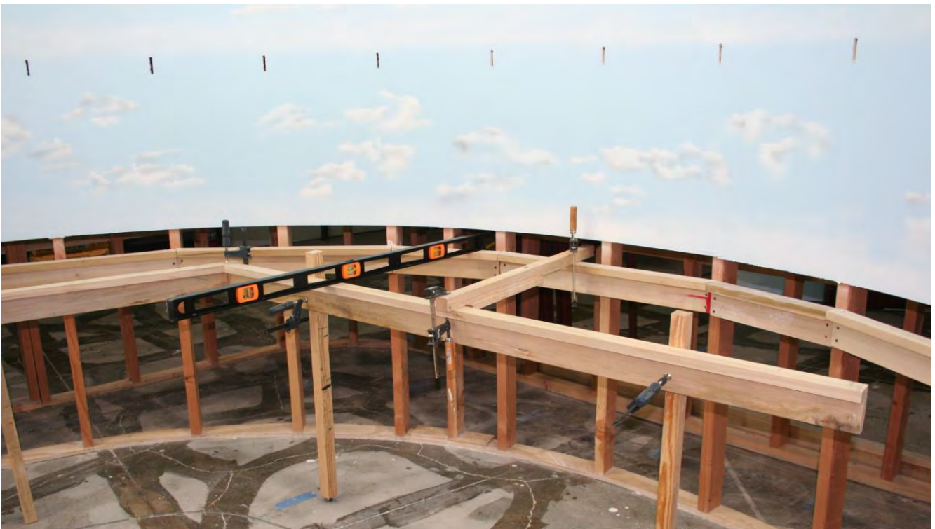
L-girder clamped in-place at Cuyler as it is being checked for level before permanent installation.
