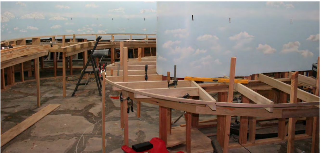
This is the end of the peninsula with the bench work now fully extended from Amarillo Junior Yard all the way thru Pampa as it stood at the end of the January 26 work day.
