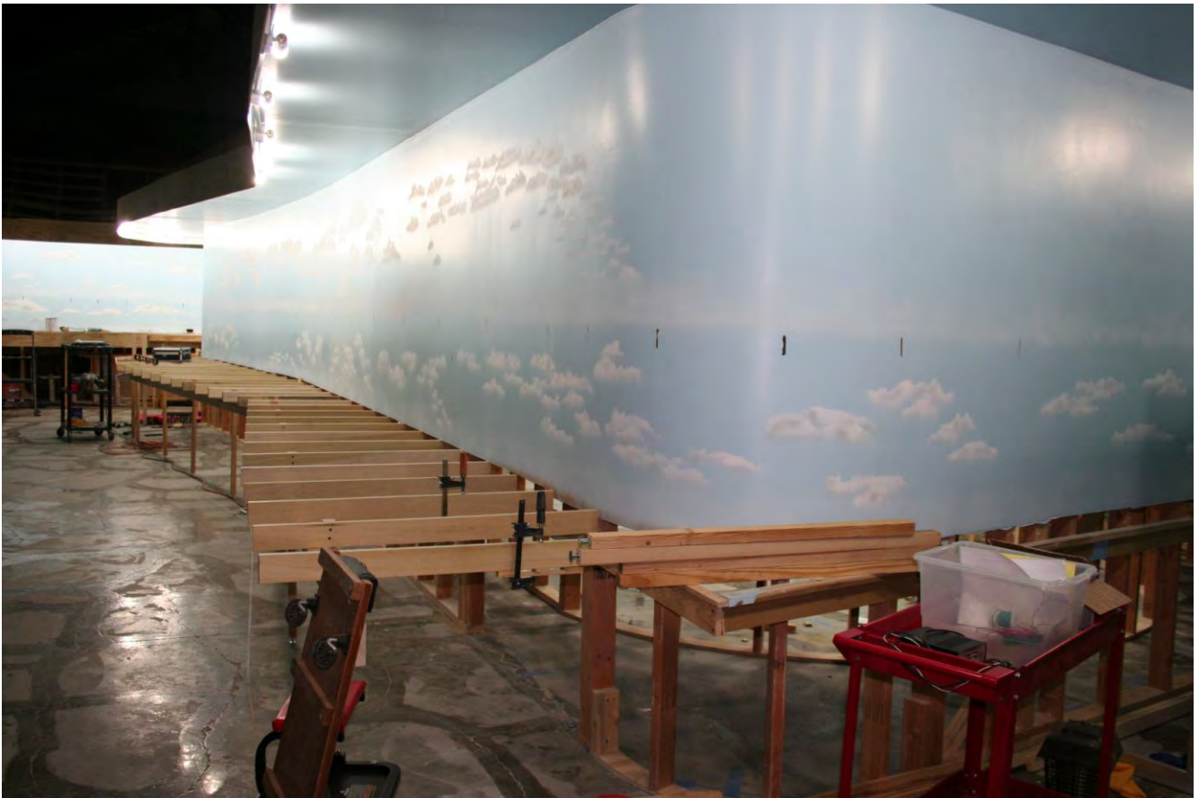
View following the end of the work day on Saturday, January 26. Joists have been installed down the full length of Pampa and the next step will be to start on the adjoining side.
