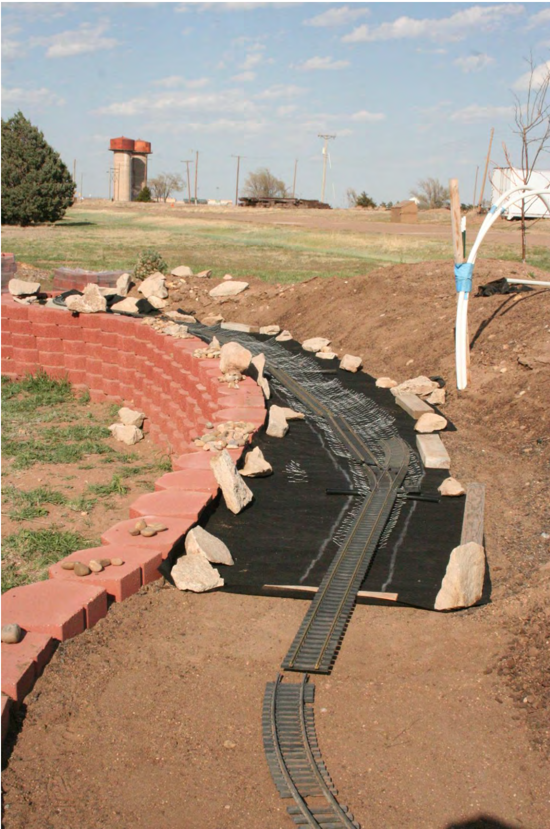
Preparations in the Phillip Pratt Memorial garden to install the track roadbed on the North side of the garden.
