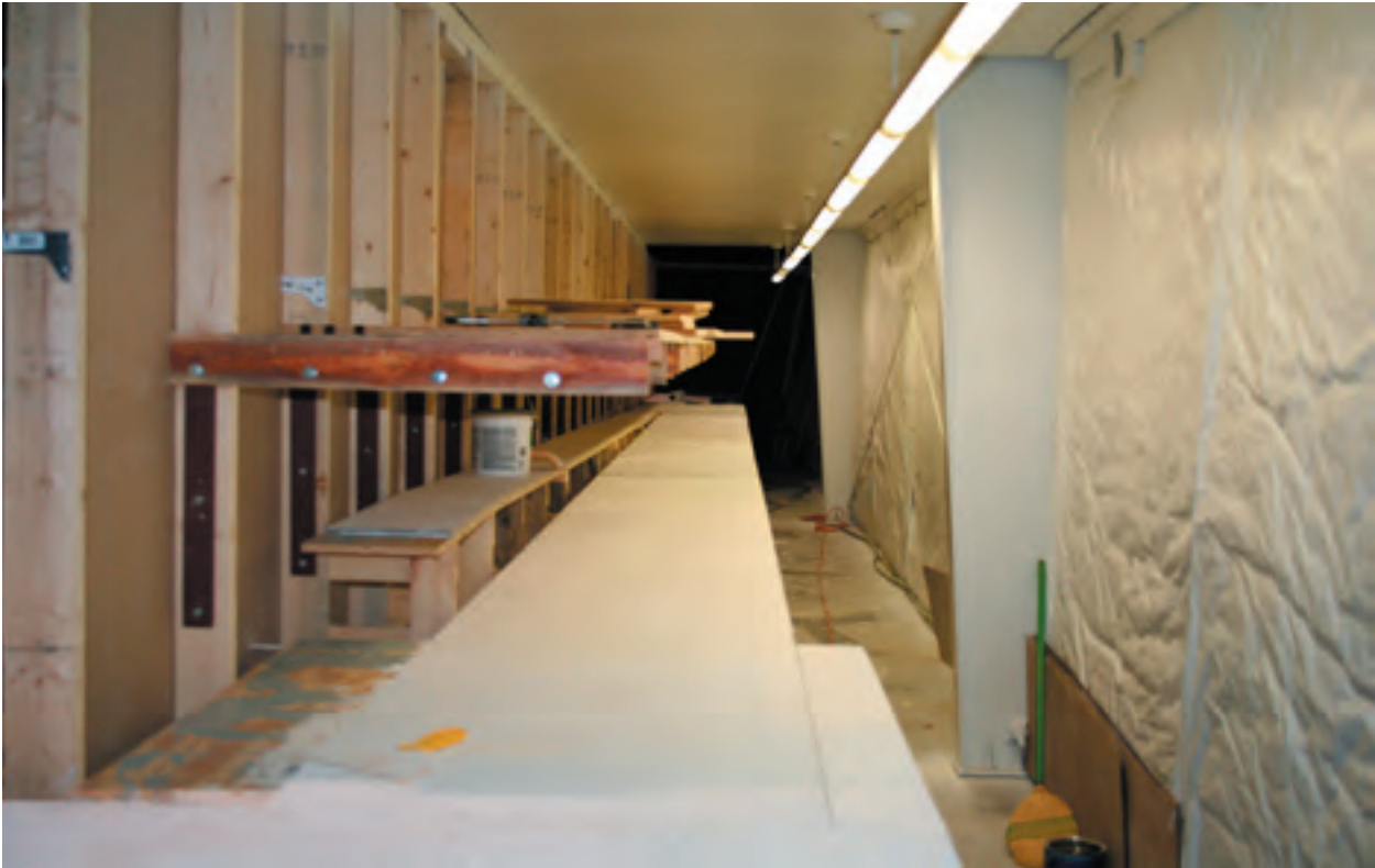
Installing the joists supporting the upper level benchwork. The L-Brackets provide no-sag support while the wood joists provide an attaching surface for the plywood above.
